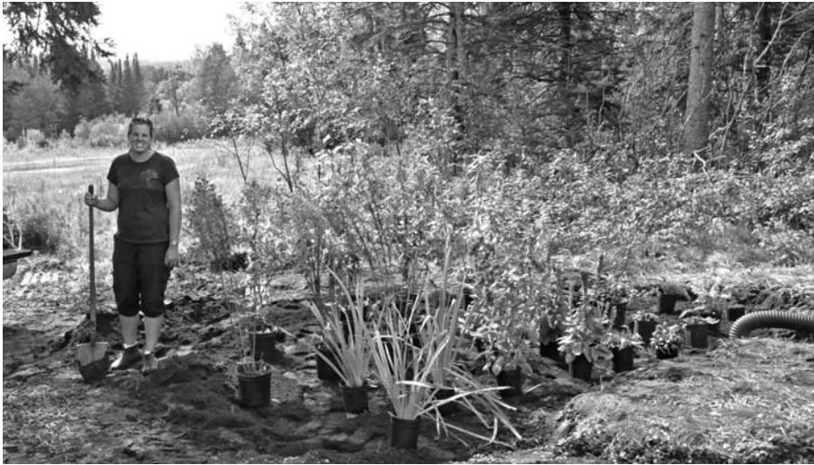
After this rain garden has been dug, a base level of gravel for increased infiltration has been added, and then topsoil added and leveled, we lay out the plants to get ready for planting.
